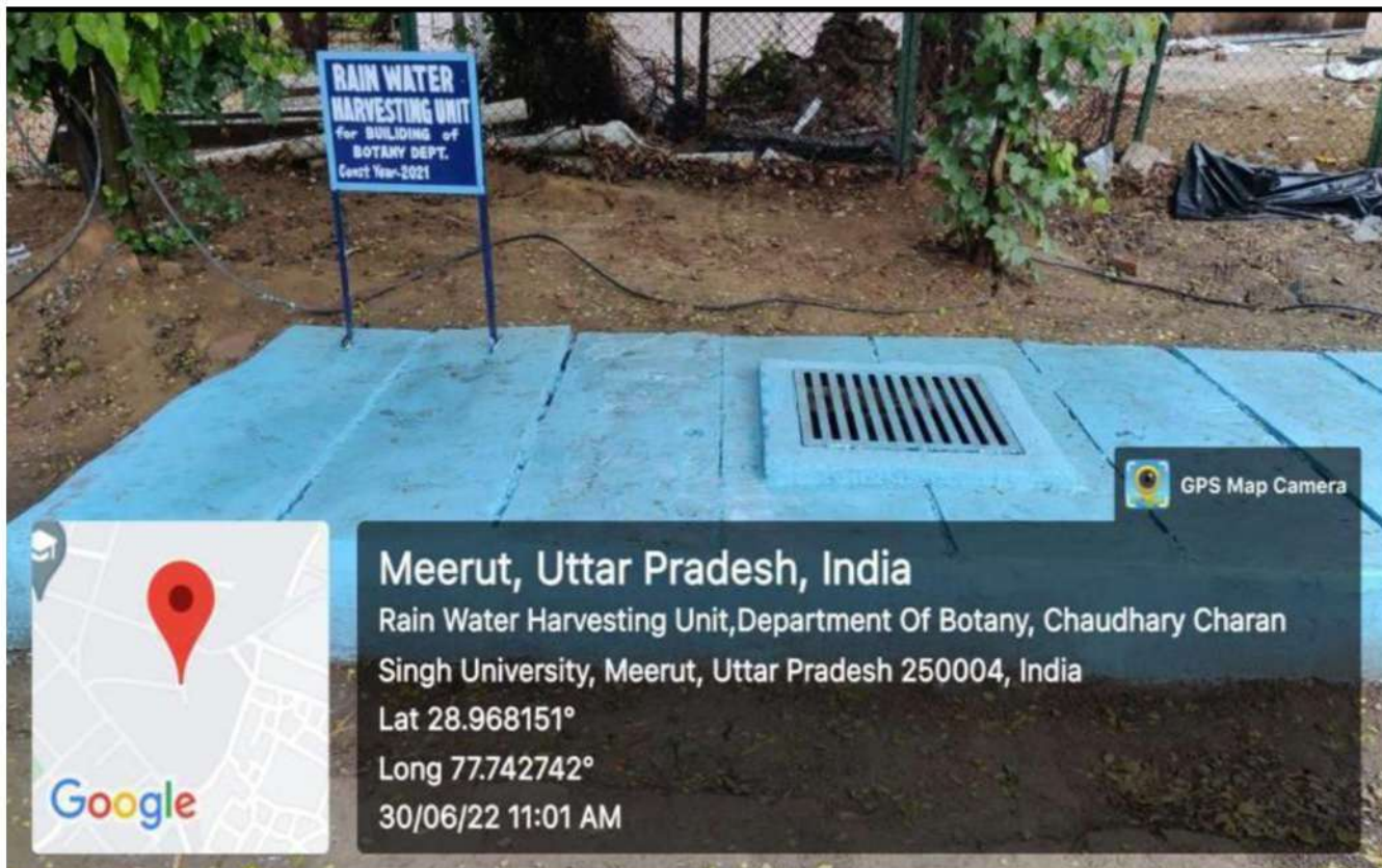
Rain Water Harvesting Units For Dept. of Botany
