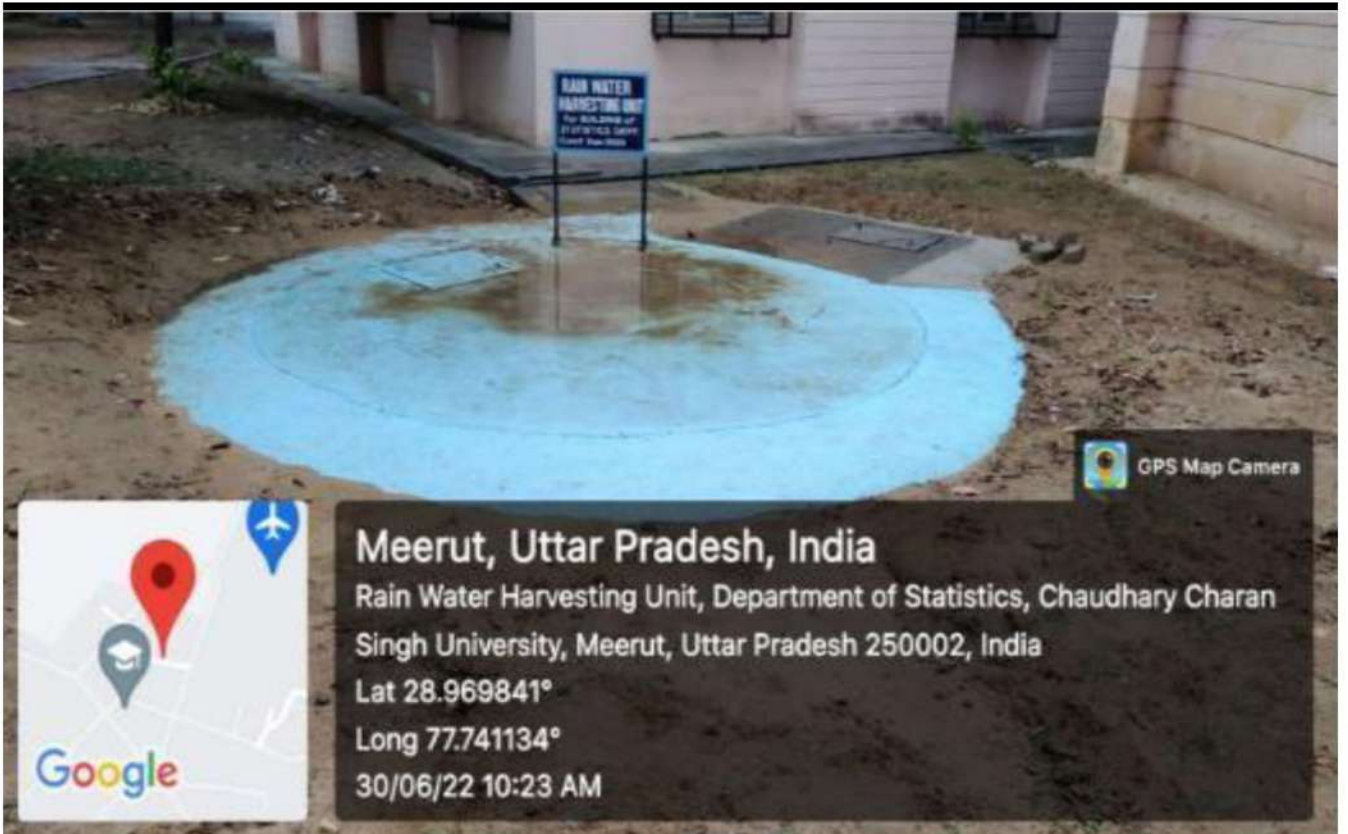
Rain Water Harvesting Units For Dept. of Statistics
