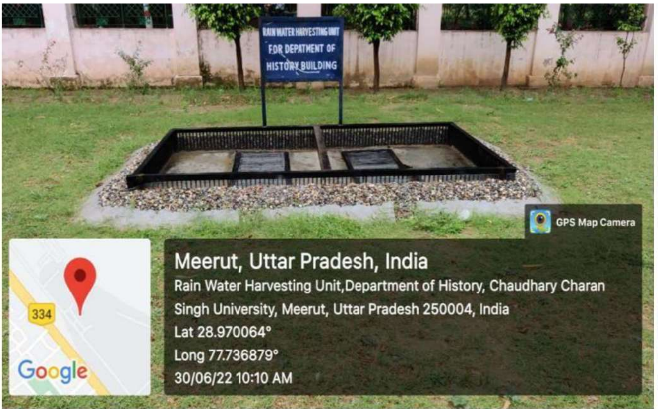
Rain Water Harvesting Unit for Dept. of History
